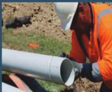
Underground Water Supply Pipeline
