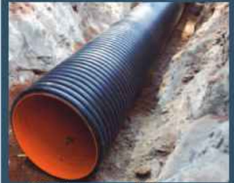
Underground Sewer Pipeline
