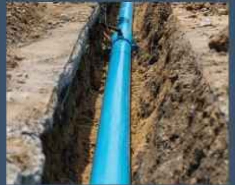
Underground Water Supply Pipeline
