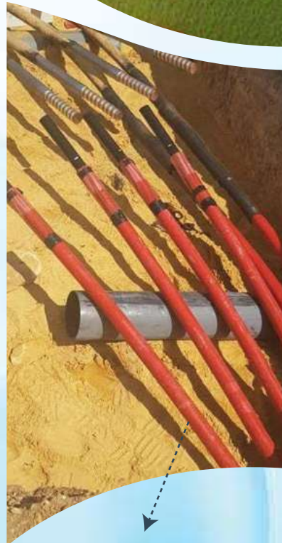
Underground Electricity Line
