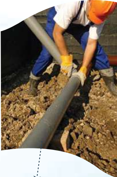
Underground Water Supply Pipeline
